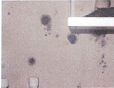
Mold on Wallboard by Hood
