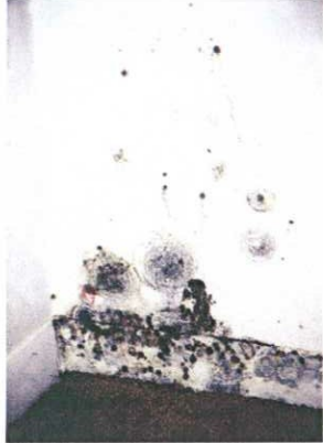
Mold on closet wallboard
