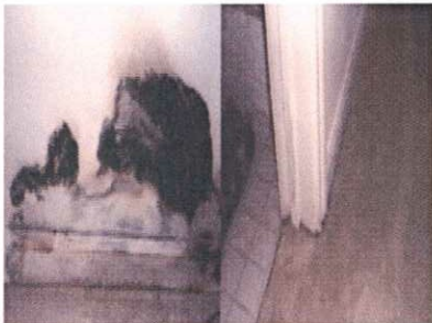
Mold coming thru wall and molding at base of door
