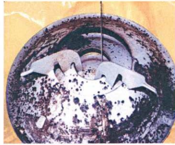
Mold on Air Diffuser
