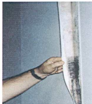
Mold Behind wallpaper with no sign on front of problem
