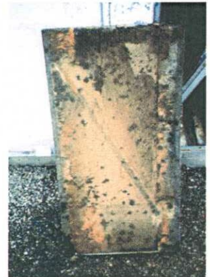
Mold on air handler panel
